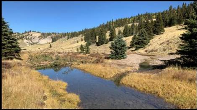
Constructed log jam on the Rio San Antonio splitting the river's flow between current channel and abandoned side channel, providing increased sinuosity and floodplain connectivity Photos by Craig Sponholz
